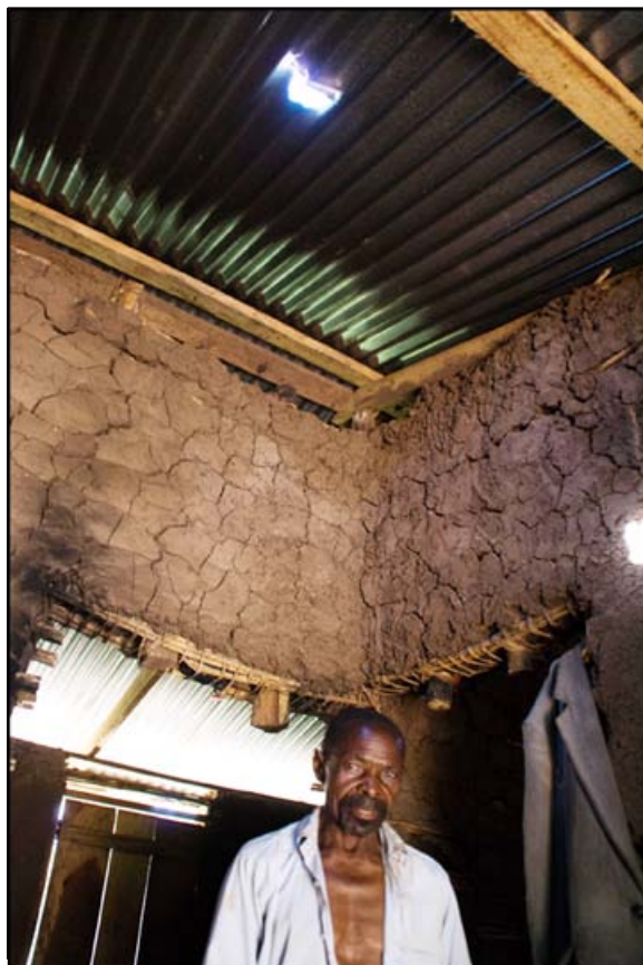
A local resident of Howa in his home situated less than 1km from the Kaiso-Tonya Road, displaying the holes in his roof and walls due to the rock blasting
